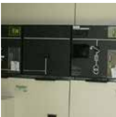
ELECTRICAL SUBSTATION TOT-2. MURCIA, SPAIN
