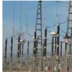
NEW SUBSTATION (66/15 KV) ANDALUSIA, SPAIN
