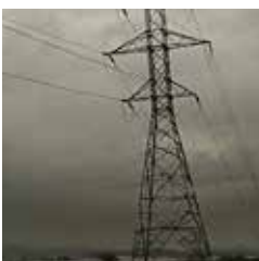
HIGH VOLTAGE LINES OF THE A-8 HIGHWAY. CANTABRIA, SPAIN
