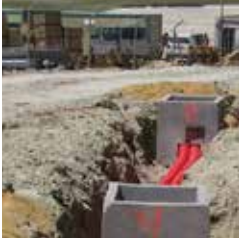
DOUBLE CIRCUIT LINE UNDERGROUND GRID CONNECTION COR I-II (15 KV) ANDALUSIA, SPAIN
