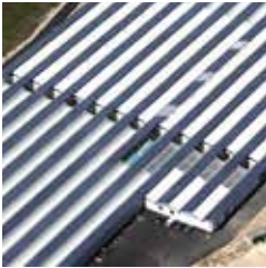
PHOTOVOLTAIC POWER STATIONS EL CORONIL (IV AND V) SOLAR GREENHOUSE. ANDALUSIA, SPAIN
