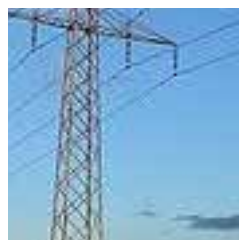
HIGH VOLTAGE LINES OF THE ANTEQUERA-GRANADA HSR. ANDALUSIA, SPAIN
