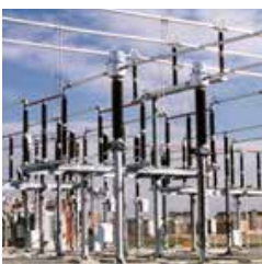
NEW SUBSTATION MAYORDOMOS (132/20 KV). MURCIA, SPAIN
