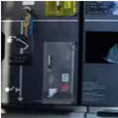
ELECTRICAL SUBSTATION CR-1. MURCIA, SPAIN
