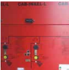
ELECTRICAL SUBSTATION CS-1 MURCIA, SPAIN
