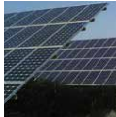
PHOTOVOLTAIC POWER STATIONS FUENTE ALAMO (I, II AND III) SOLAR FARM IN MURCIA, SPAIN
