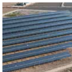
PHOTOVOLTAIC POWER STATIONS IN 6 SOLAR GREENHOUSE. TOTANA. MURCIA, SPAIN
