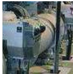
NEW SUBSTATION LAS AGUILAS-GUADELESTÍN (132/20/6,3 KV) MURCIA, SPAIN
